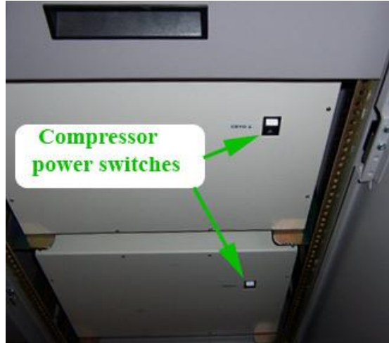
Figure 29 - MX Series compressor power switches
